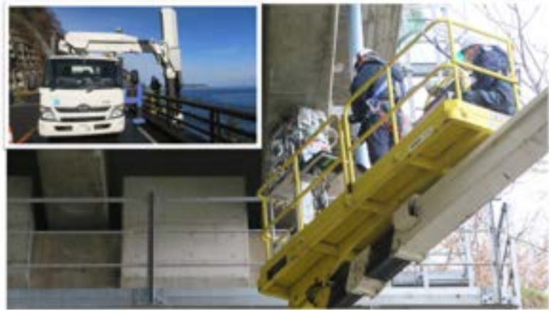
図2 実橋梁でのRANS- \mu 計測の様子。左上：橋梁上から見た橋梁点検車 右：橋梁点検車バケット様子 Fig.2: RANS- \mu measurement on a real bridge. Top left: Bridge inspection vehicle seen from the bridge top Right: Salt-density measurement by RANS- \mu installed in the bucket
